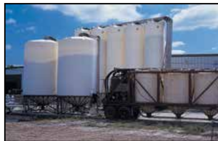
Large cone bottom tanks ranging in sizes from 2,500 to 13,000 gallons, are used to store and deliver up to 10,000 cubic ft. of bulk resins at a processing plant.
